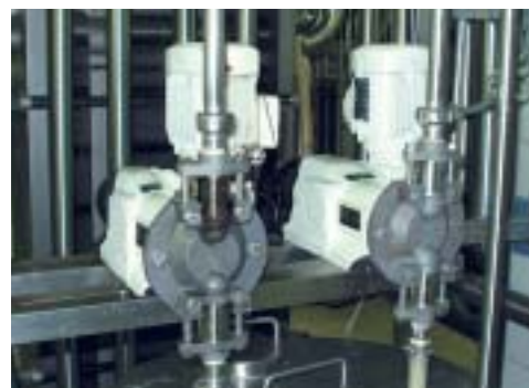
Two Préci Pump Lagoa Series pumps in the dairy industry: pumps with stainless steel body for dosing acid and soda in the Cleaning In Place zone
