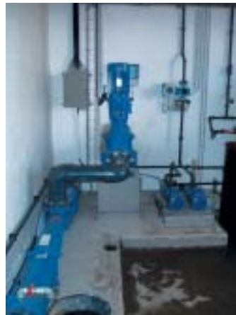
Feeding of dehydration equipment
