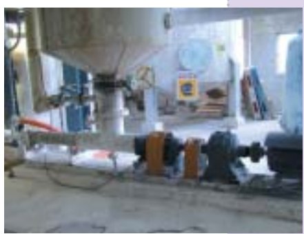
IVA pump for transfer of silica
