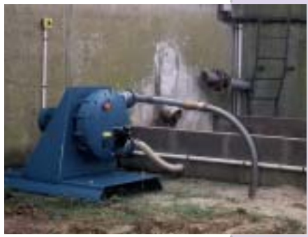
DL pump for recovery of spume and floating matter on decanter
