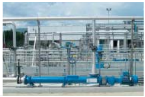
I pump for lime milk dosing
