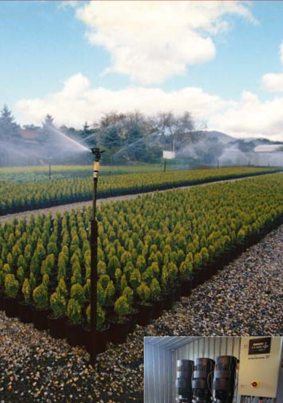
Grundfos Hydro 2000 booster in irrigation system at Humphris Nursery, Australia, boosting the pressure of water for the production of camellias.
