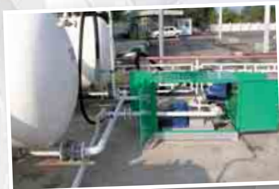
Aboveground autogas installation using one autogas series pump with three tanks.
