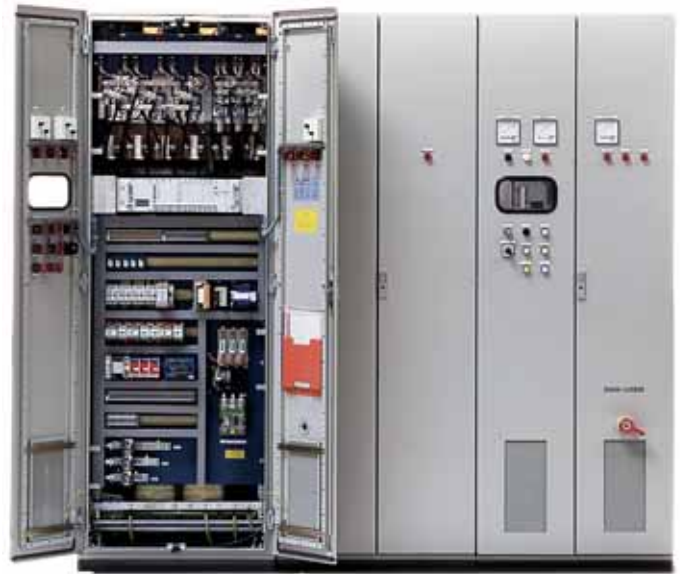
Example of control cabinet
