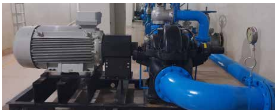
NR. 2 SKDZ-4P 200-630 400kW VIETNAM HYDRAULIC POWER STATION
