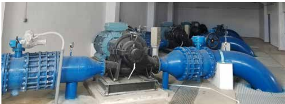
NR. 4 SKDZ-4P 200-630 400kW ALGERIA DRINKING WATER SUPPLY
