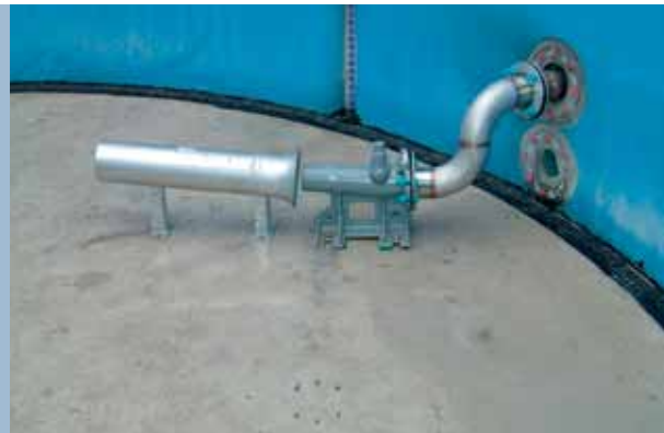
Inside the tank: The nozzle and ejector pipe are located to generate a bulk flow loop, which leads to re-suspension and homogenization of the mixed sludge.
