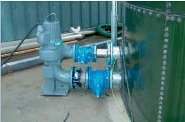
Outside the tank: The Flygt jet mixer N-pump. Stainless steel pipework is fitted to the tanks for suction and delivery.
