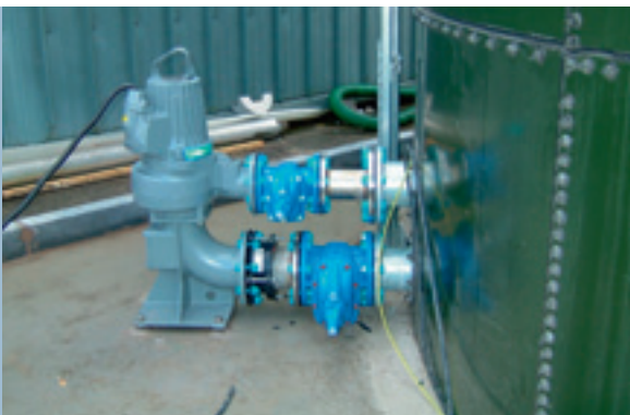
Outside the tank: The Flygt jet mixer N-pump. Stainless steel pipework is fitted to the tanks for suction and delivery.
