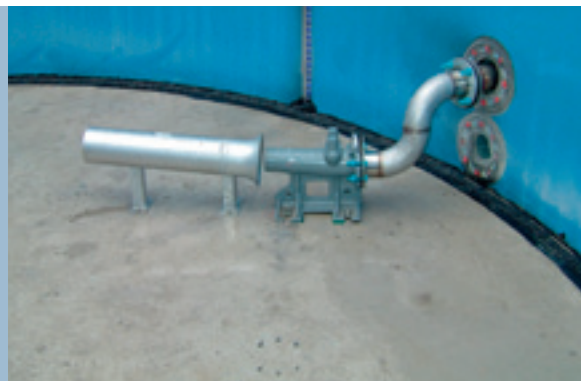
Inside the tank: The nozzle and ejector pipe are located to generate a bulk flow loop, which leads to re-suspension and homogenization of the mixed sludge.
