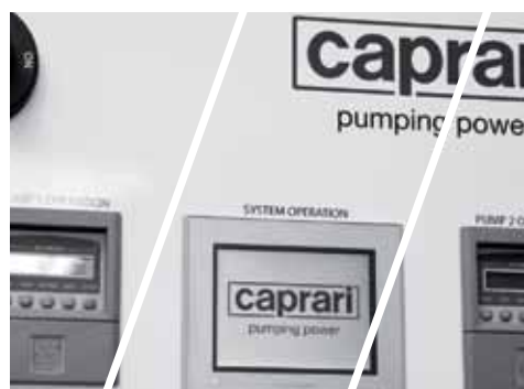
Pump Control Technology
