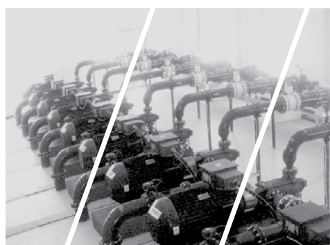
Boosting and Distribution of surface water
