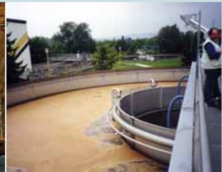
Wastewater Treatment Plant Aeration Tank (Tank in Tank) Diameter: 20.20 m Height: 4.50 m
