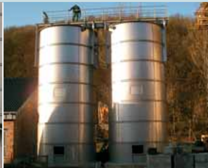
Sludge Storage Tank with Access Platform Diameter: 4.63 m Height: 10.50 m
