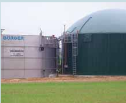
Biogas Plant Digester and Storage Tank Diameter: 18.53 m / 16.67 m Height: 6.00 m / 6.00 m
