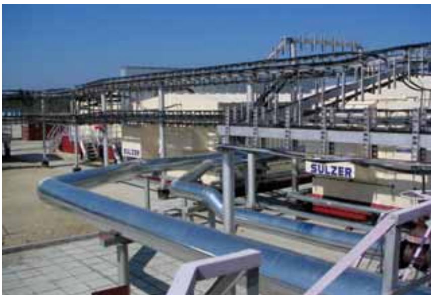
Pumping station in Western Siberia: three MPPs operating in parallel.
