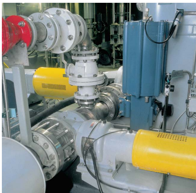
Fig. 29. ClO 2 mixing with chemical mixer.
