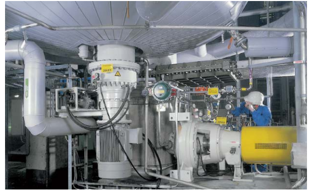
Fig. 17. MC® tower discharge pumping system.
