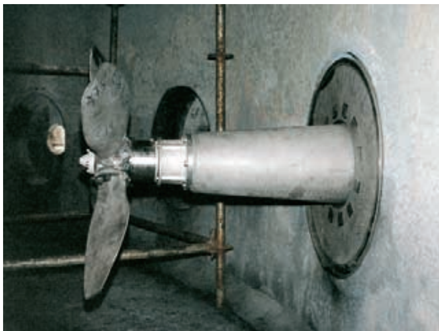
Fig. 3. A modern SALOMIX™ agitator with a 30 kW motor and 1000 mm propeller. This agitator was mounted into a 1200 m 3 Green Liquor Stabilization Tank in February 1997, and it alone has replaced the three agitators shown in Figure 2.
