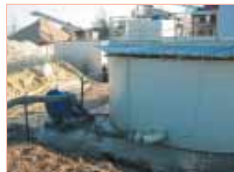
Filter press feeding in a quarry
