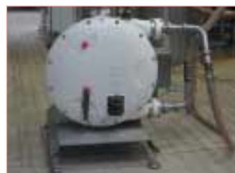
Tomato pulp transfer from storage to preparation tank
