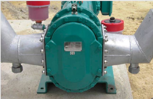
Feed pump for a biogas substrate. Flow rate up to 40 m 3 /h at a pressure of 2 bar.
