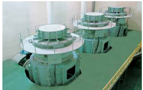
Dock Dewatering Pump
