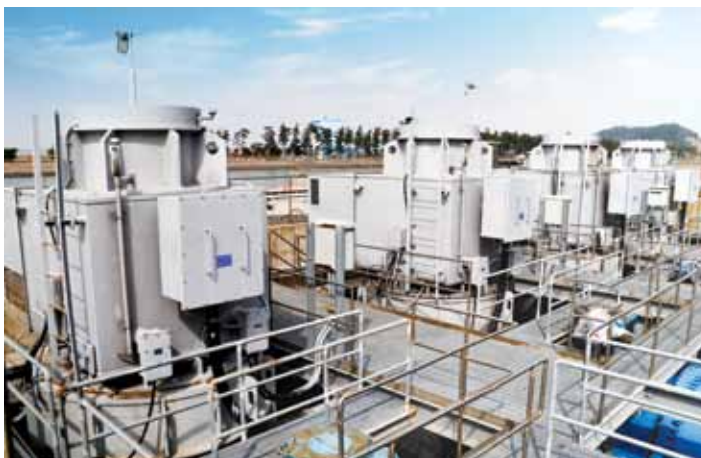
Circulating Water Pump for Taeon Thermal Power Plant
