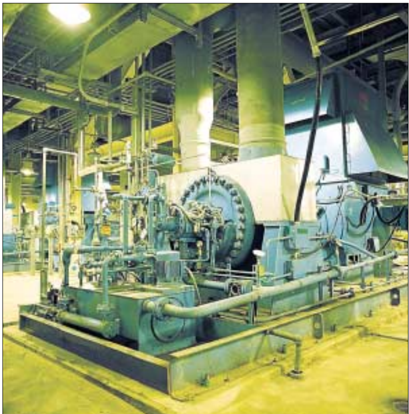
Feedwater booster pump for Yonggwang Nuclear Power Plant, unit 3 & 4, Korea (Model 600 × 400HDM)
