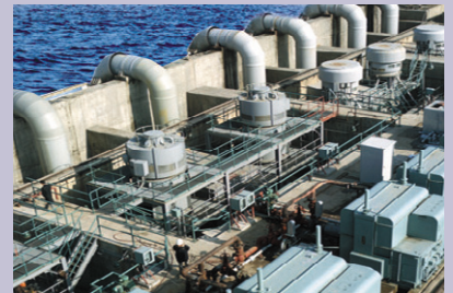
Sea Water Lift Pump for Thermal Power Station 2000VKNM
