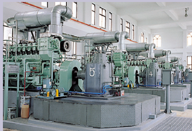
Drainage Pump for Drainage Station
