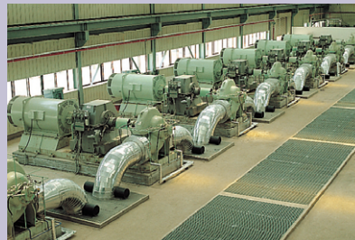
Hot Water Supply Pump for Bundang Model 600 X 400HDM
