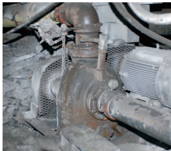
Self-priming centrifugal pump in a mine.
